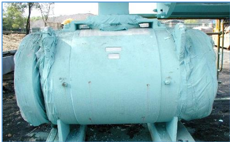
Valve body after wet application. Note, the nameplate and data plate have been left uncovered. They were later covered by removable PFP access panels.
