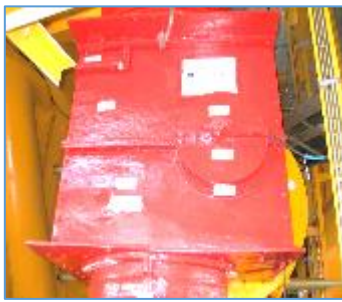
Completed 36" Main SDV, installed and fitted with its PFP castings and wet applied PFP.
