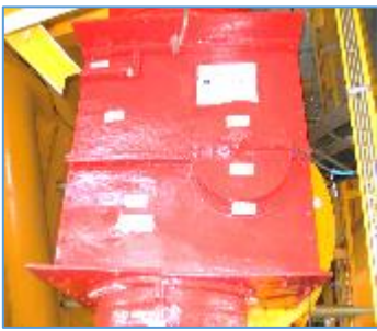
Completed 36" Main SDV, installed and fitted with its PFP castings and wet applied PFP .
